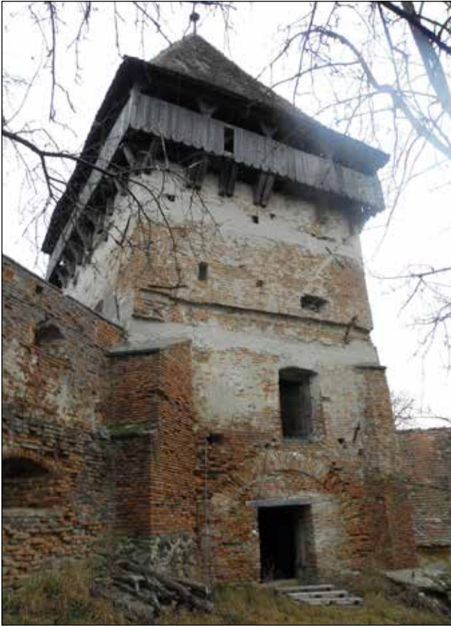
■ Foto 3. Alma Vii, Turnul Slăninii înainte de restaurare © MET ■ Photo 3. Alma Vii, Larder Tower before conservation © MET
